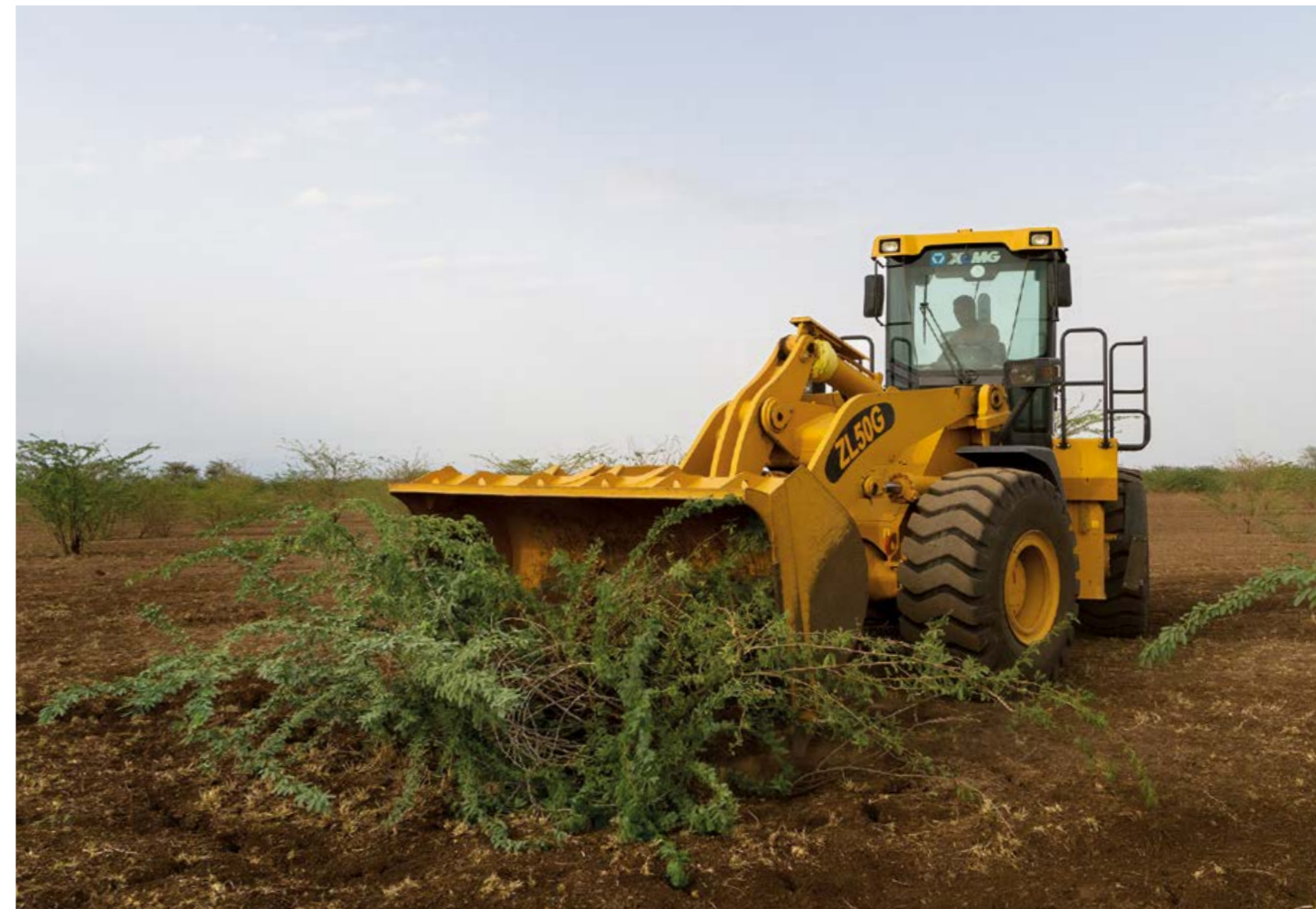
A bulldozer clears the rangeland near the community of Halaydege, in Amibara woreda, Afar of prosopis juliflora by pulling it up from the roots “We could not have cleared in two months what the (PRIME) project’s loaders did in three days,” says community elder Ahmed Birigo. “Now it is our responsibility to be sure the rangeland is not re-invaded.”
