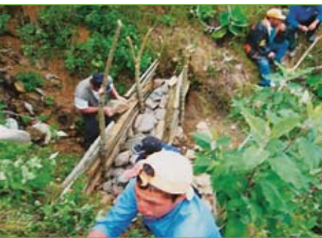
Implementing erosion control measures resulting from land use planning in Guatemala (see A2)
