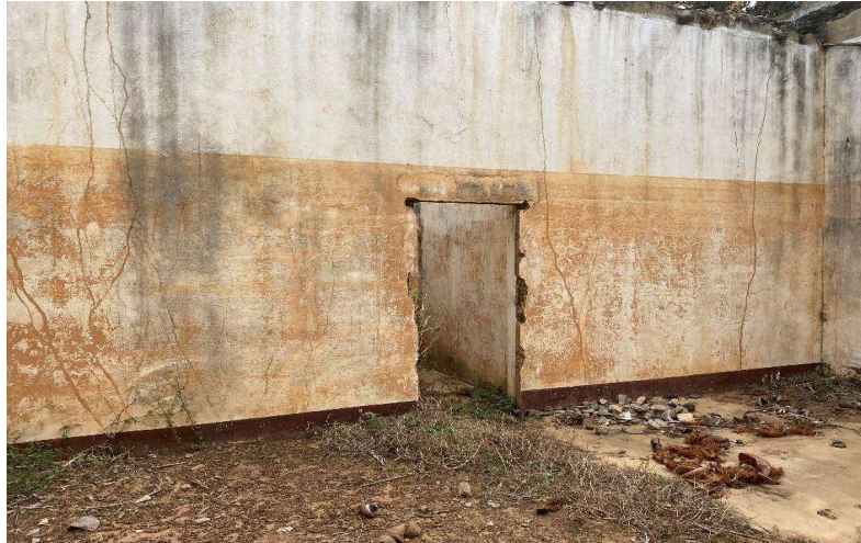
Figure 11: Photo of an abandoned house showing marks left by flood waters
