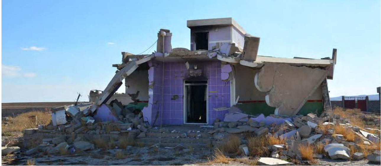
Many well-built houses, like this one in Sinuini, have been reduced to rubble by the fighting. Photo: UN-Habitat
