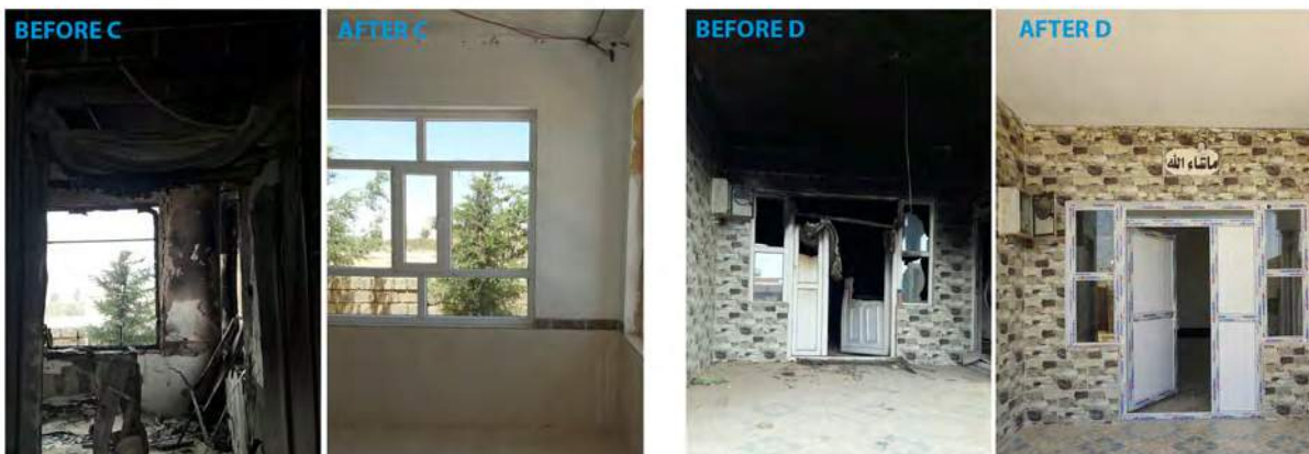
Before and after rehabilitation: Efforts in Sinjar to restore housing to its rightful occupants and rehabilitate it. Photo: UN-Habitat
